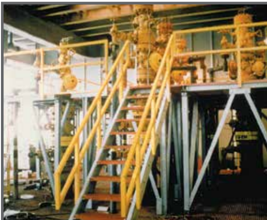
Dynaform support structure and square tube railing provide a high level of corrosion resistance for this offshore platform.
